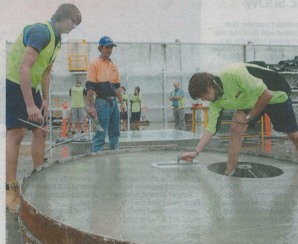
HARD WORK: Year 11 students from Kawana Waters State College get working at Tellam Civil Products at Warana last week. PHOTO: NICHOLAS FALCONER/SCN23021TELLAM
